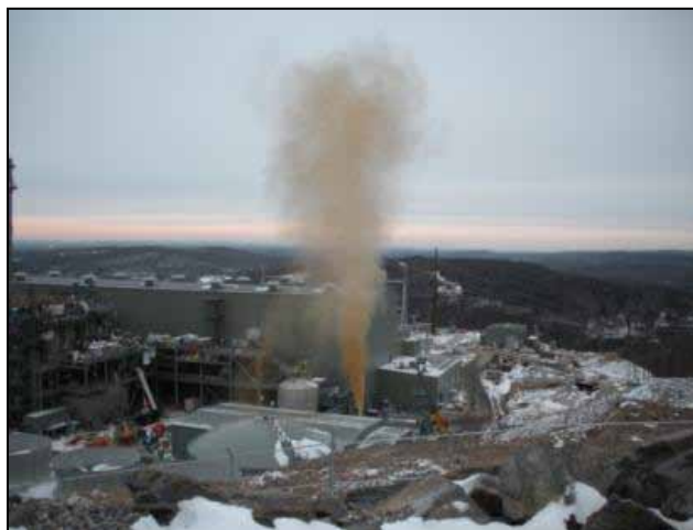
Figure 4-1 Iron Oxide and Debris Coming from Pipe
