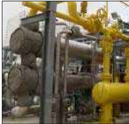
Figure 2-9 Typical Shell and Tube Heater for Heating Natural Gas to Meet Turbine Performance Requirements
