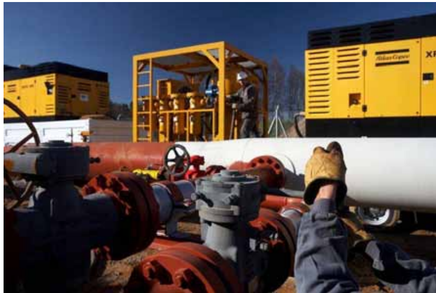
Figure 8-2 Typical Rental Screw Compressors Installed at a Job Site
