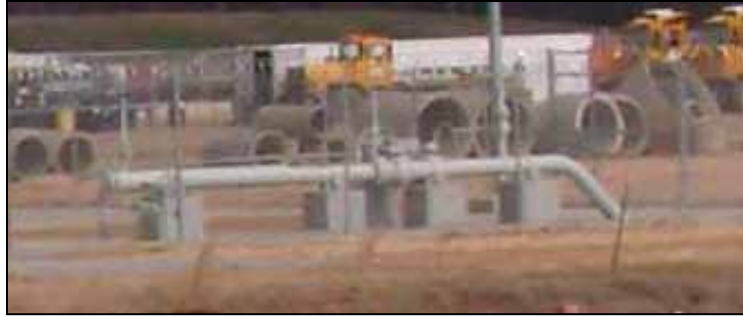
Figure 2-4 Gas Yard Pigging Station Receiver/Launcher
