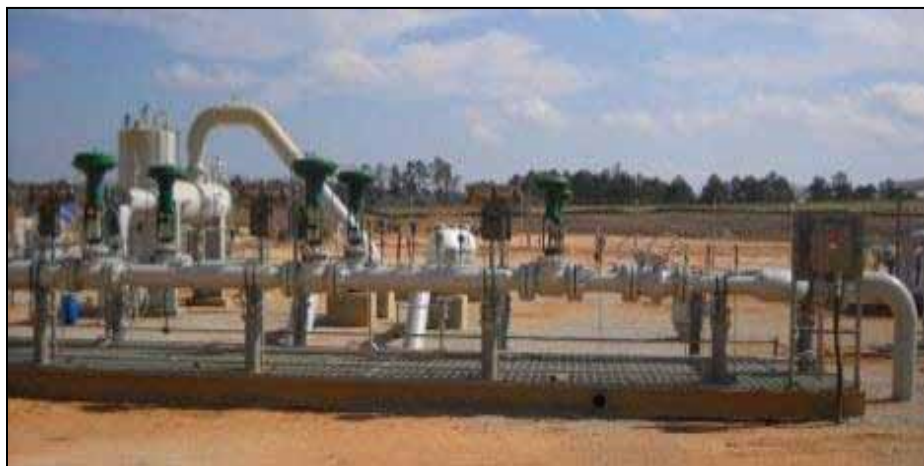
Figure 2-5 Typical Gas Yard Pressure Regulators
