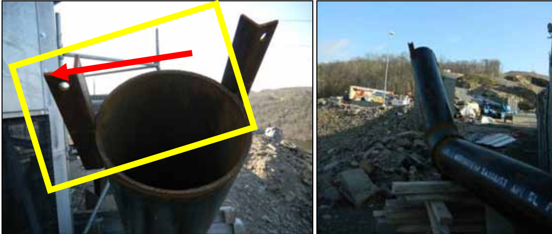
Figure 5-1 Temporary Piping for Pipe Pneumatic Blow Cleaning Discharge with Target Mounting Bracket and Outline of Where a Target Would Be Mounted
