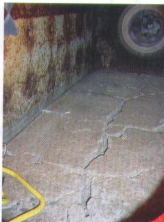
Fig 3 Example of refractory failure resulting from thermal shock due to unexpected fast shutdown
