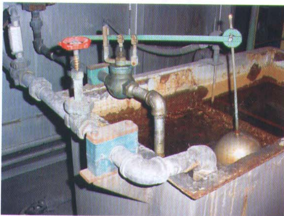
Fig 2 Open cooling system that supplies water to door seals. A furnace cooling system is critical to safe operation.
