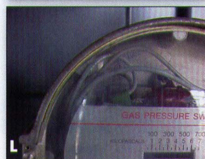
PHOTOS K and L. Setpoints that are obviously wrong.
