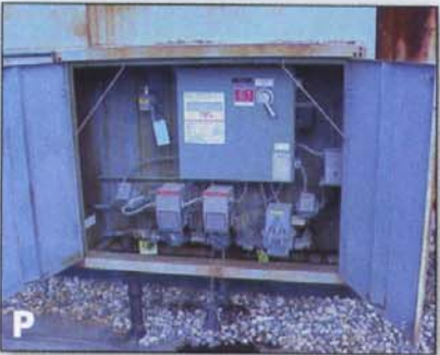
PHOTOS N, O and P. Automatic valve actuator failures can make for downtime and hazardous operating conditions.
