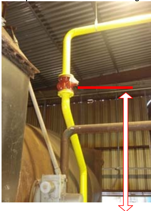
Example Manual Shutoff Valve Too High
